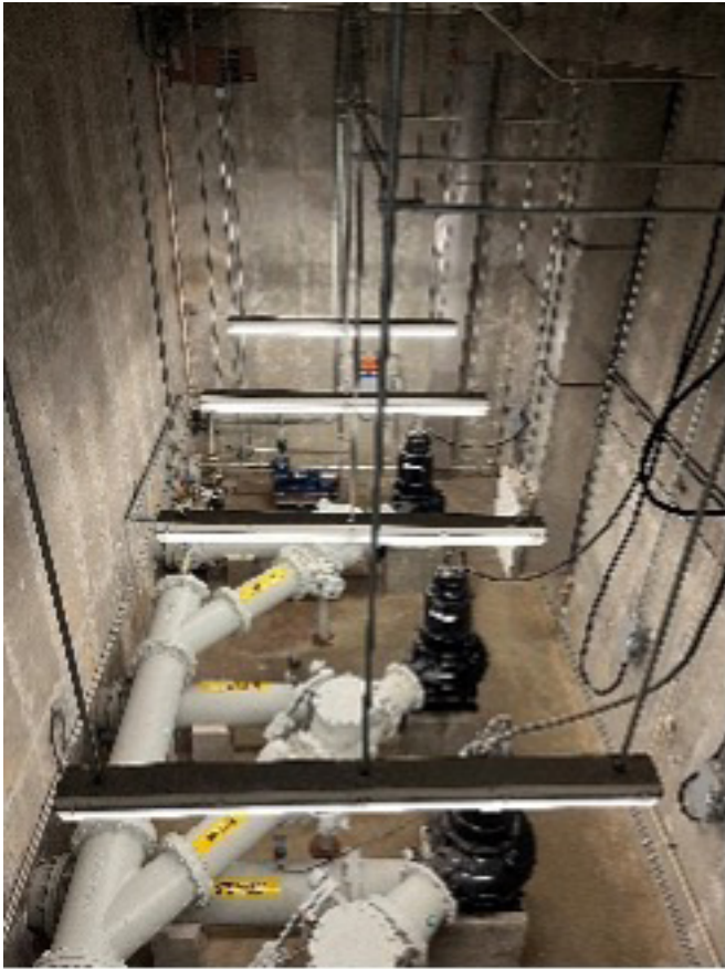
Photos (above and previous page) from the Essex Junction Wastewater Plant
